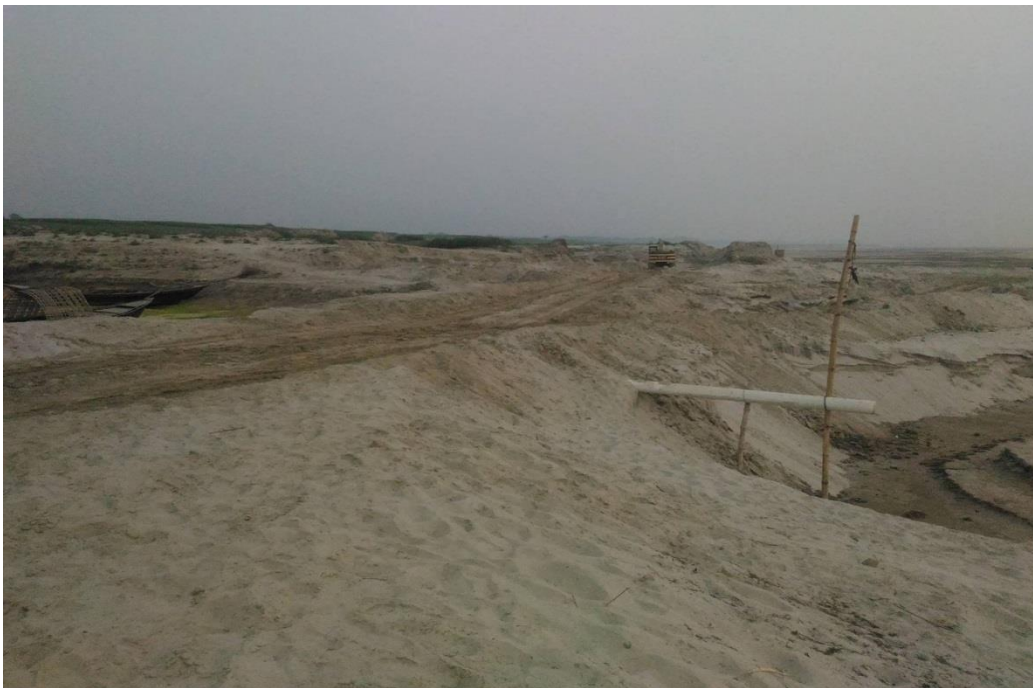
FIGURE S2 The sand-mud barrier built across the Baral River (right of image) to facilitate sand mining from the Padma River (top left of image)
