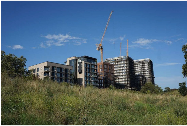
Figure 3. New-builds in construction on Site 1a of the Aylesbury Estate redevelopment in August 2023. Author's photograph.
