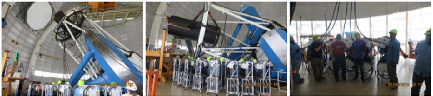
Figure 41. The fiber cables and slits were stored on their shipping carts during the focal plane installation and handled by an expert team of NOIRlab engineers during cable routing. The middle and right panels show the NOIRLab team, each person managing one fiber cable and spectrograph spool box with slitheads as the fiber cables are installed to the telescope.
