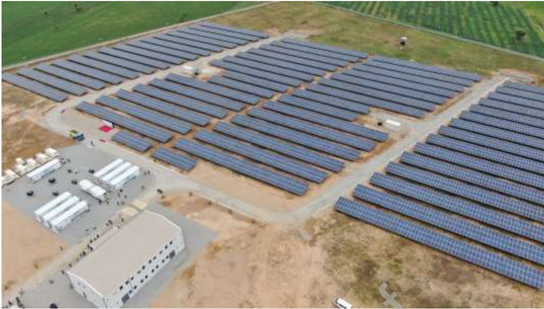
Figure 1: EEP solar hybrid power plant at Bayero University, Kano state (REA, 2019)
