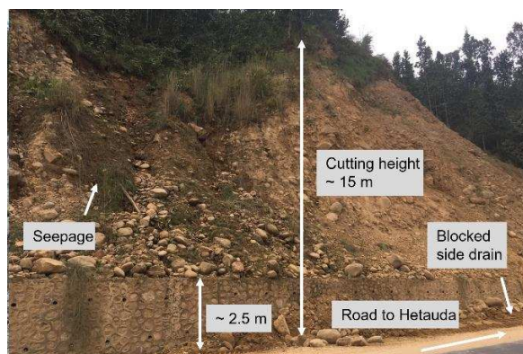
Figure 4: Example of an ineffective mortared masonry wall on the Madan Bhandari Road.
