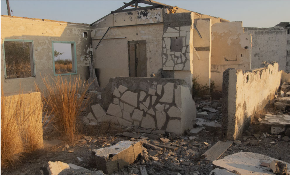
Figure 5. The Richmond school in July 2019, after its demolition by SBA authorities, following negotiations on the MoU.
