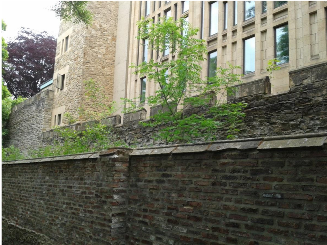
Figure 6: View of the Castle Wall beside the Pace Building, with the wall of the Bishops' Walk in the foreground and showing how the Castle wall follows the change in ground level within the wall.
