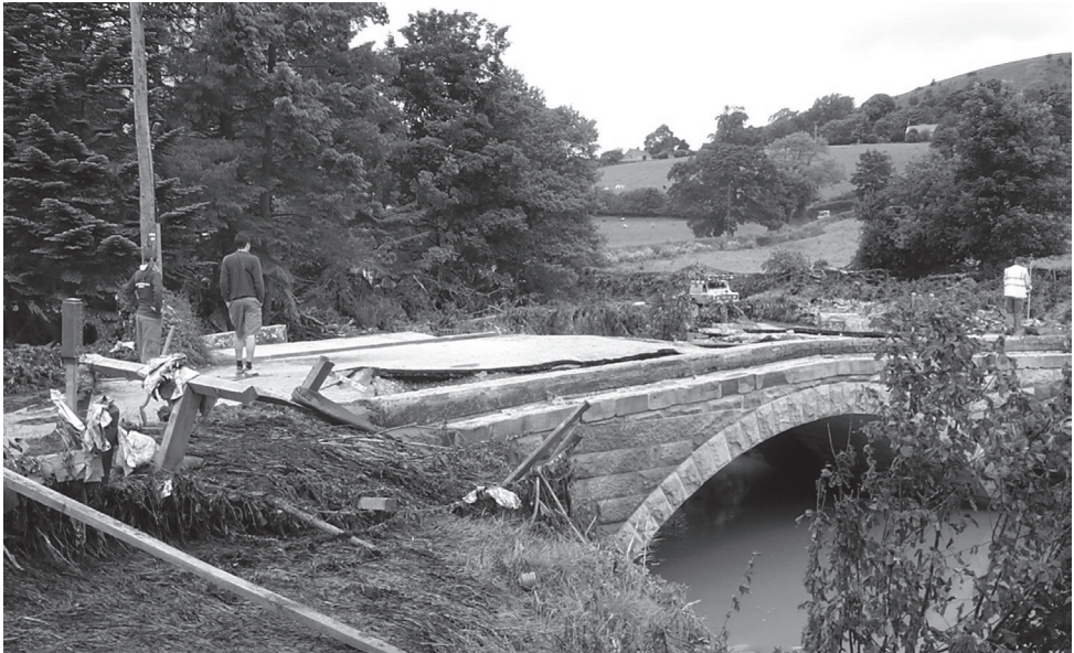
Figure 2. Flood damage at Hawnby
