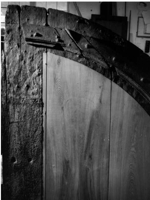
Figure 4: Upper front face of the West Leaf of the North Door during restoration. Photographed in raking light by Trevor Woods, Department of Archaeology, University of Durham. Note the corroded nailshanks and raised ridges of the original strapwork
