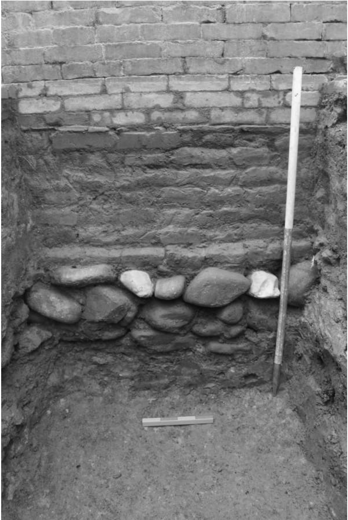
Figure 11: Stone cobble and brick foundations of Char Narayan Temple in Trench 1C.
