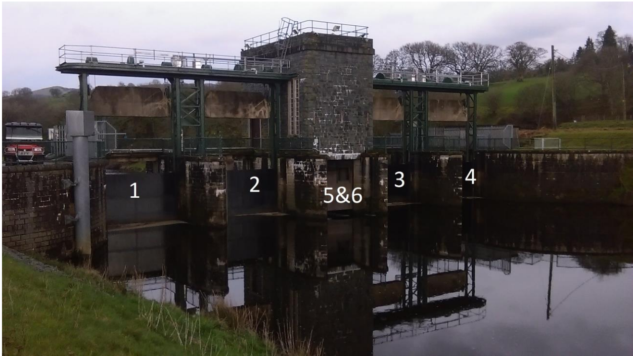
Figure 2. Bala (Llyn Tegid) sluices, sluice gates are numbered from the left 1, 2, 5, 6 (hidden behind 5), 3 and 4. Photograph taken during springtime water level retention, guillotine gates 1-4 are undershot passage routes and as can be seen gate 5 is lifted clear of the water presenting a central surface orientated passage route.
