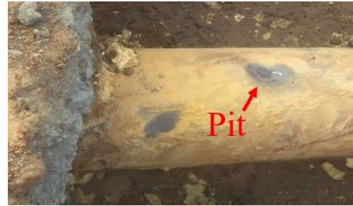
Fig. 14: The photo of found pit in pipeline.
