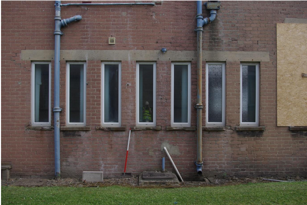
Fig 15 The lavatory windows in the west elevation of the office block of K51. Although these differ from the four large windows shown on the building control plan (TWAM CB.GA/BC/plan/NET/52) the surrounding brickwork shows no sign that they were added later and so are probably part of the original build.
