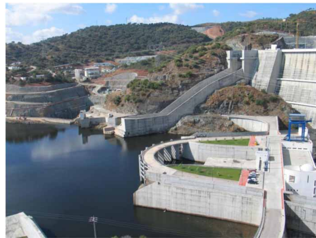
Figure 3 | The Alqueve Dam, on the Guadiana River in southern Portugal, has created Europe's largest reservoir. Photo Veronica Strang.
