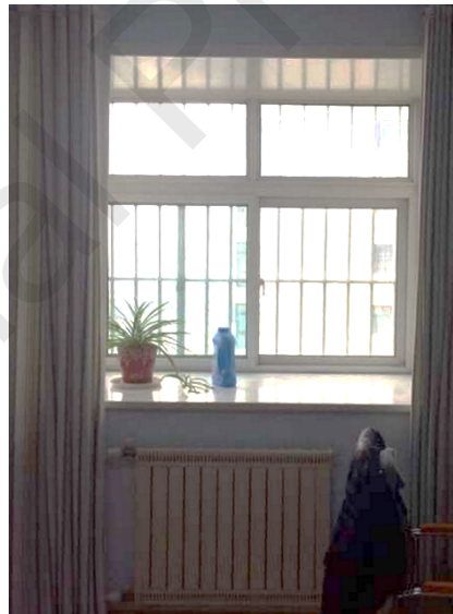
Figure 4: The radiator for room heating.
