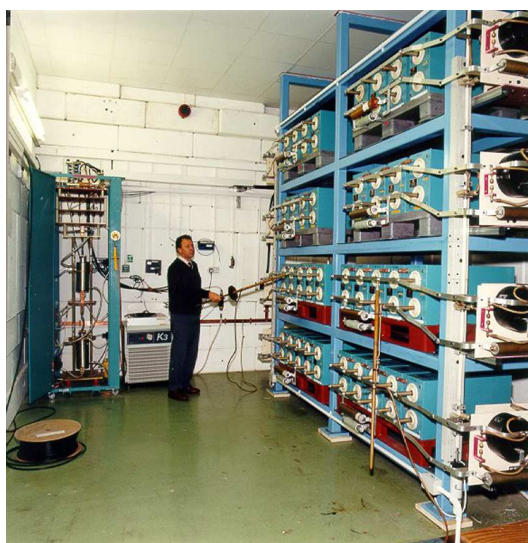
Figure 66. The CLF's Ray Wyatt inside the VULCAN capacitor bank showing ignitrons in the left cabinet and HVR resistors in the main circuit. (Picture courtesy of STFC.)
