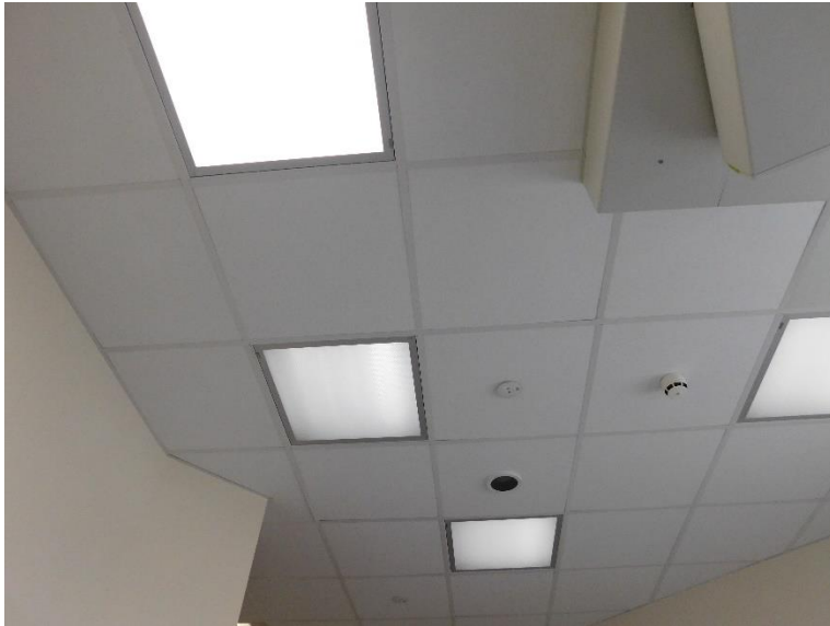
Figure 2. View of the ceiling, from the patients position in a critical care side room
