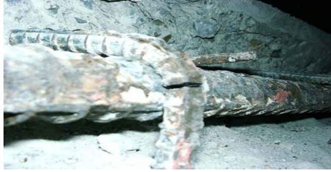
Fig. 1: Example of fractured steel bar.
